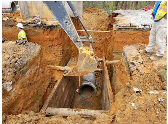
Above: A project to repair stormwater drainage along Woodway Road earlier this year.
