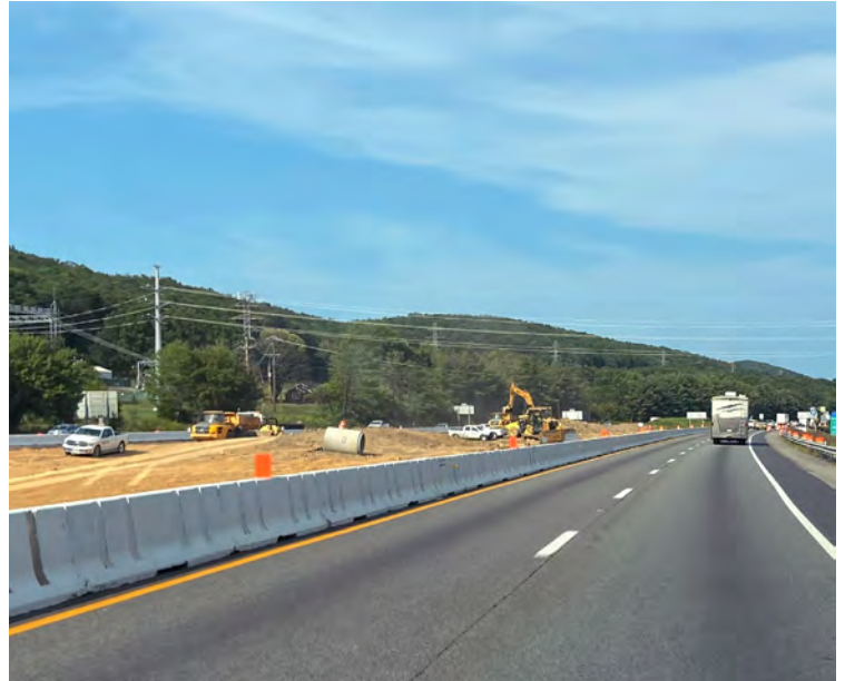
Above: The project to widen I-81 between exits 141 and 143 is expected to be completed in 2022.
