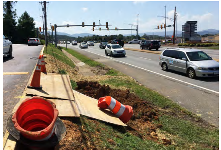
Above: Construction on Electric Road / Route 419 in front of Tanglewood Mall. Completion of this project is anticipated for November 2021.
