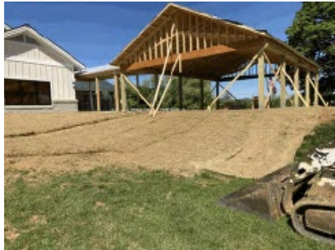
Properly installed and maintained erosion and sediment controls have been consistently used at the Saint Francis Service Dogs Pavilion project.
